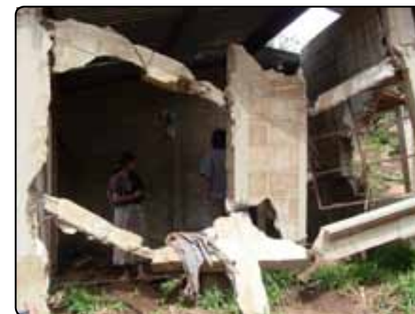
The remains of a house in the village of San Juan, Comalapa.
